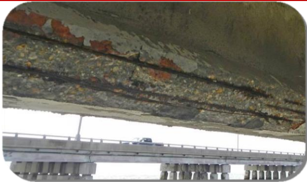
Poor (Structurally Deficient)
