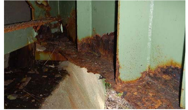
Poor (Structurally Deficient)
