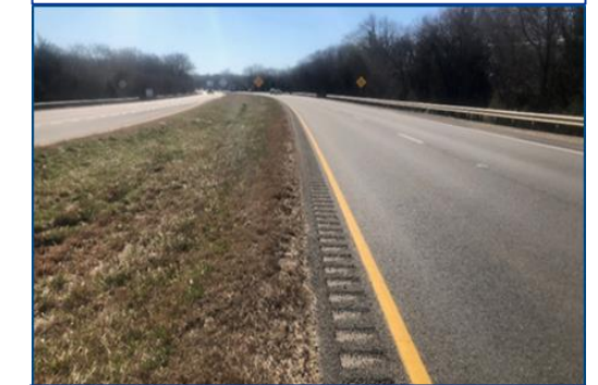
Edgeline Rumble Strips
