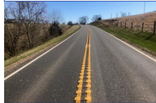
Centerline Rumble Strips
