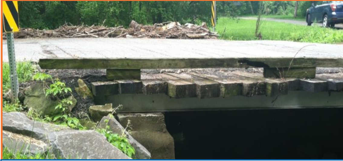
14 Ton Posting – Loudon County Prohibited Garbage Pickup Service
