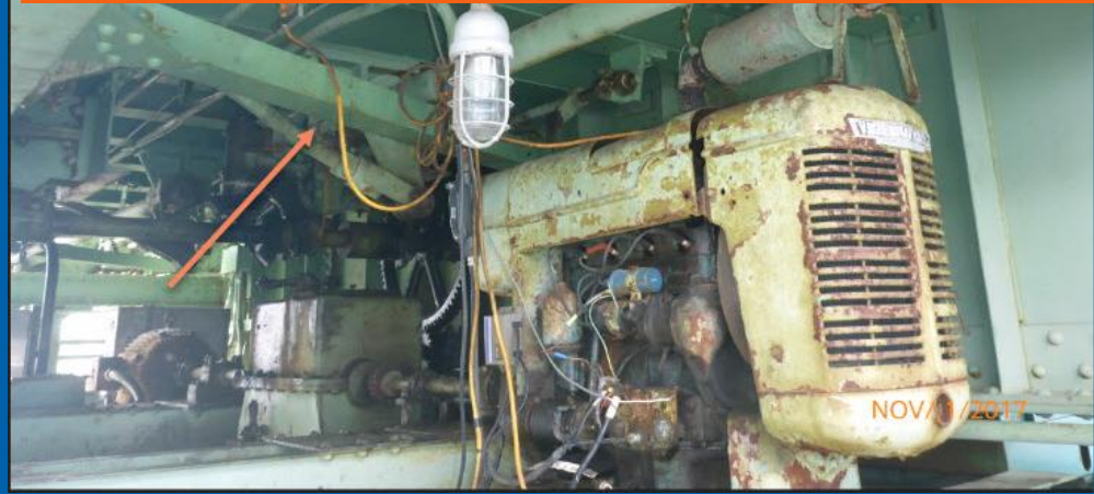
Gwynn's Island Aging Generator
